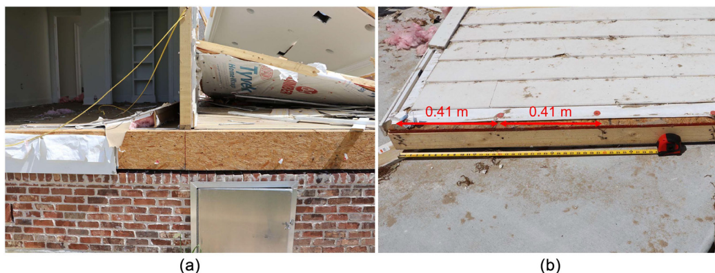
Fig. 9. Local wall structure failures due to a discontinuity in the structural load path at the wall's bottom plate to floor connection caused by (a) wall sheathing not overlapping the join, and thus (b) sole reliance on the limited lateral capacity of the nailed connection between the bottom plate and floor structure. (Images by David B. Roueche.)
