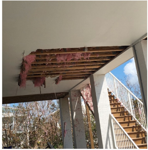
(b) Hurricane Irma
