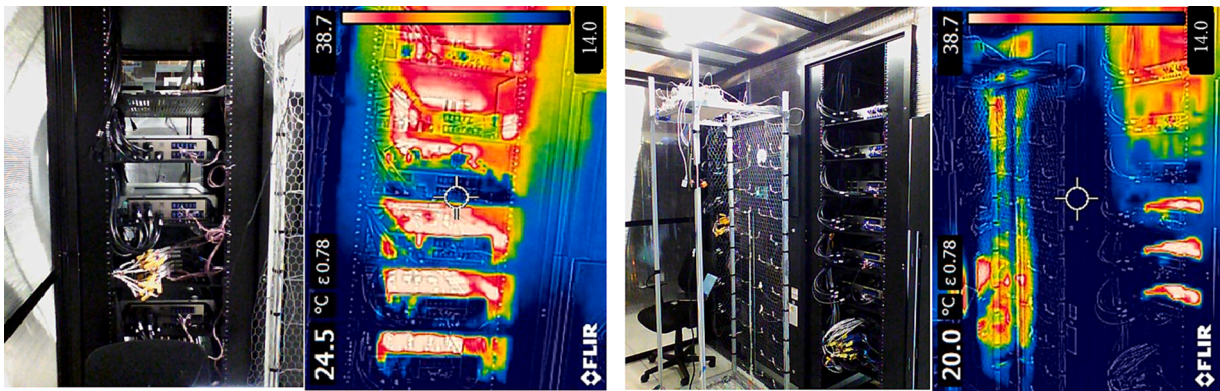
Fig. 10. IR images taken during the experiment in the cold aisle before installing the blanking panels.
