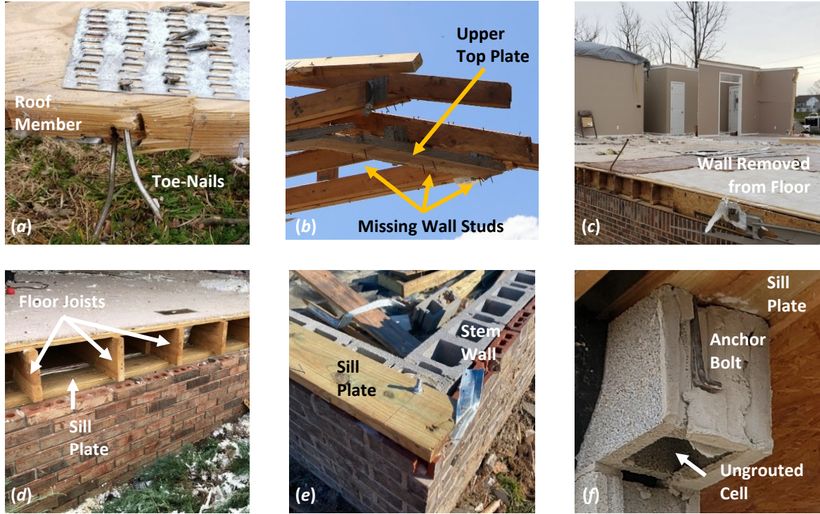
Figure 2. Post-storm damage observations involving (a) toe-nailed roof-to-wall connection failure, (b) stud wall failure, (c) removal of wall framing from floor framing, (d) loss of rim joist, (e) failure of floor joist to sill plate connection, and (f) partial collapse of concrete masonry stem wall.
