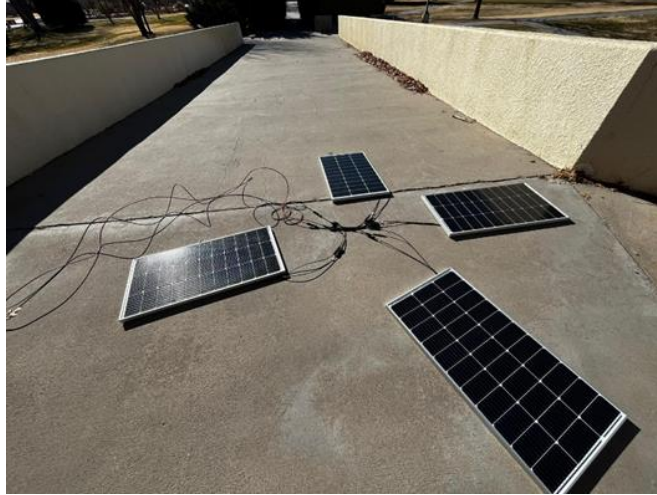
Fig 3. The orientation of the solar panels
