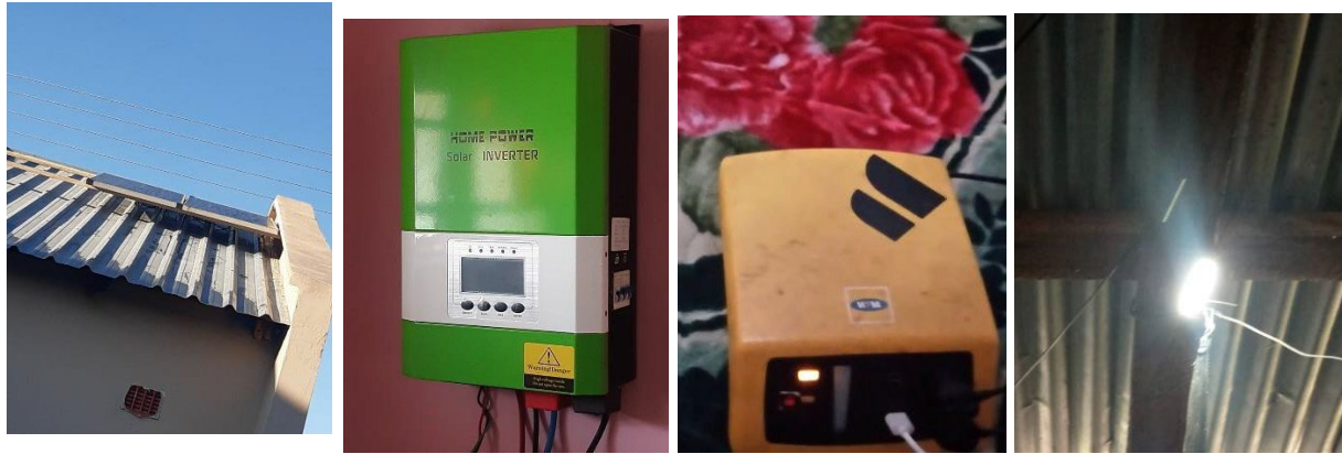
Figure 3 (Left to right): Rooftop solar panels, solar inverter, solar prepaid system, solar lights. Photo credit: Enumerators
