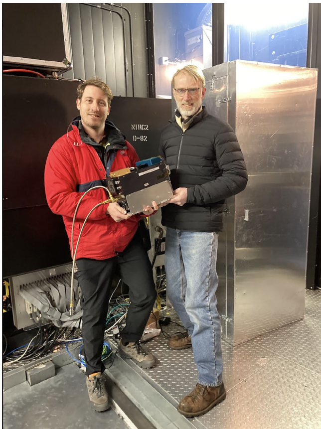
FIGURE 1 Timothee Greffe and David Hale from Caltech delivering the new controller. Behind them is the NIRC2 instrument (D-82 dewar) and the 6-ft tall electronics cabinet that the new controller replaces.
