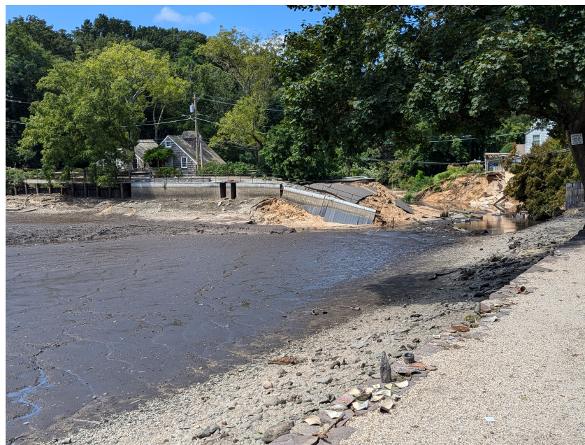
Figure 2. View to the site of the collapsed Harbor Road in Stony Brook.
