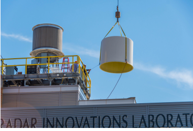
Fig. 1. The CPPAR installed at the rooftop of the Radar Innovations Laboratory at the University of Oklahoma.
