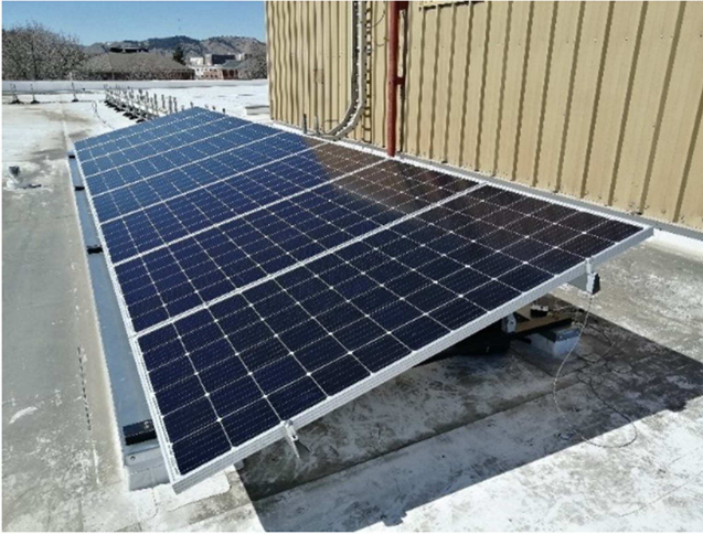
Fig. 1. 3-kW grid-tied PV system on campus.
