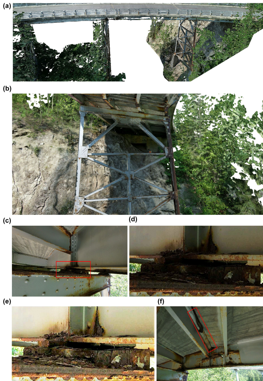
Figure 8. Canyon Creek Pedestrian Bridge condition assessments: (a) 3D model viewed from the northeast direction, (b) 3D model viewed from underneath the fourth span, (c) bearing condition, (d) close-up view of the bearing, (e) enhanced image, and (f) joint sealant condition.
