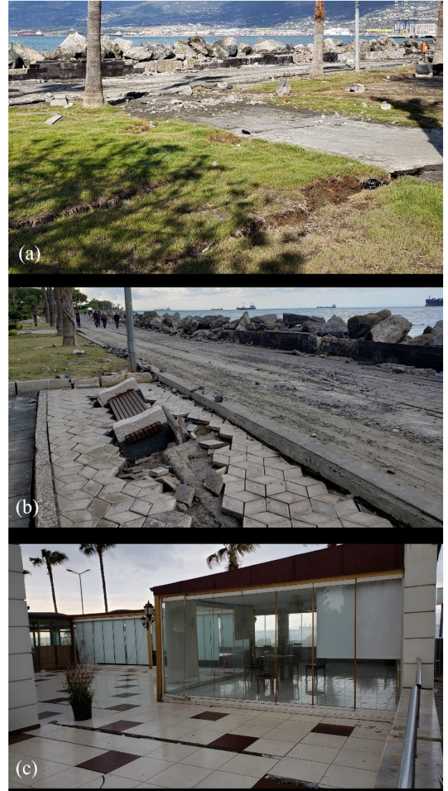
Fig. 5. Lateral spreading damage observed on April 1, 2023: (a) park area along transect LS-4 (36.5930N, 36.1687E); (b) sunken park bench and ground deformation behind Doğan restaurant patio (36.5937N, E36.1672E), and (c) cracking in patio along back of Doğan restaurant building (36.5935N, 36.1671E)
