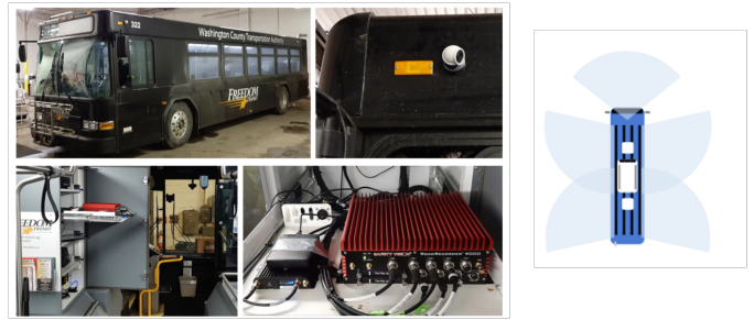
Fig. 4: The left four images show the commuter bus, an image of the computer, the cabinet that contains the computer and electronics, and one of the cameras. The right diagram shows the field of view of each installed camera, where one faces forward and four side cameras face opposite directions from each other.
