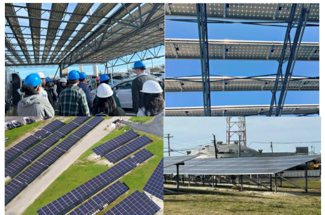
Fig 2. Solar installations in ACUA's Solar Array Project [8].
