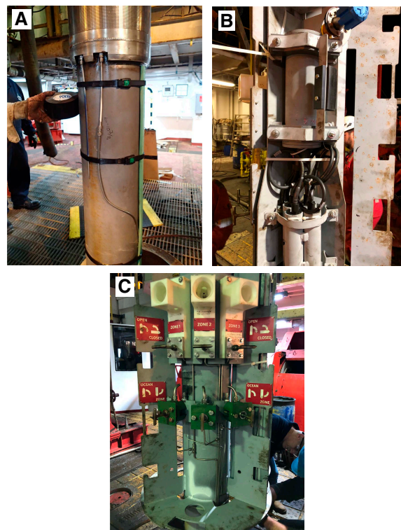
Figure F62. Pressure sensing components, Hole U1518H. A. Pressure monitoring screen (above) and umbilical pressure lines strapped to ACORK casing. B. Pressure monitoring data logger and pressure gauges on ACORK wellhead. C. Valves and external sampling ports connected to pressure umbilicals on ACORK wellhead.
