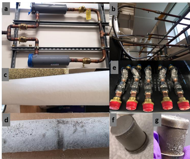
FIGURE 3: (a) Supply manifold 25-micron filter driers with replaceable cores. (b) Row manifold looped to itself by hoses. (c) New filter. (d) The filter after flushing. (e) Manifolds with 40-micron filters are used to loop the rack with itself. (f) New filter. (g) The filter after flushing.
