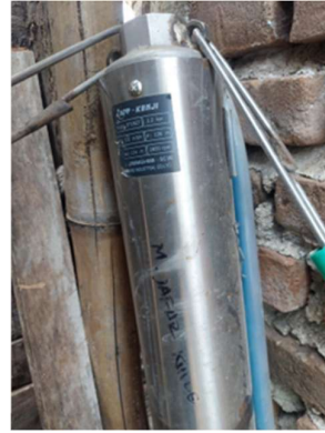
Figure 4. Installed water pump.
